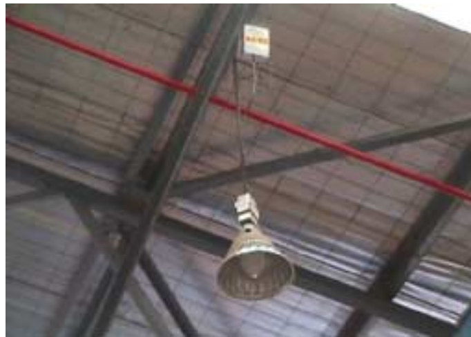
Relay box attached to metal halide lamp fitting.
