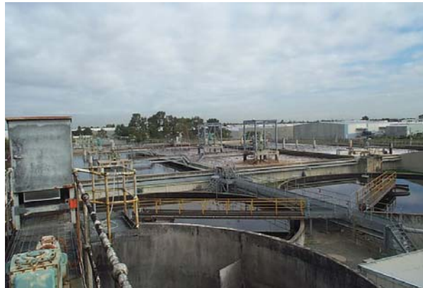
Wastewater treatment plant
