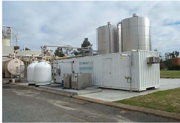
Reverse osmosis treatment plant
