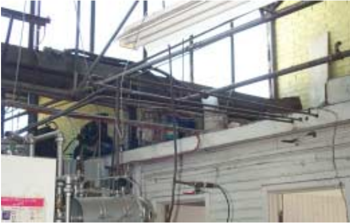
At the previous premises steam pipes were uninsulated and very long.
